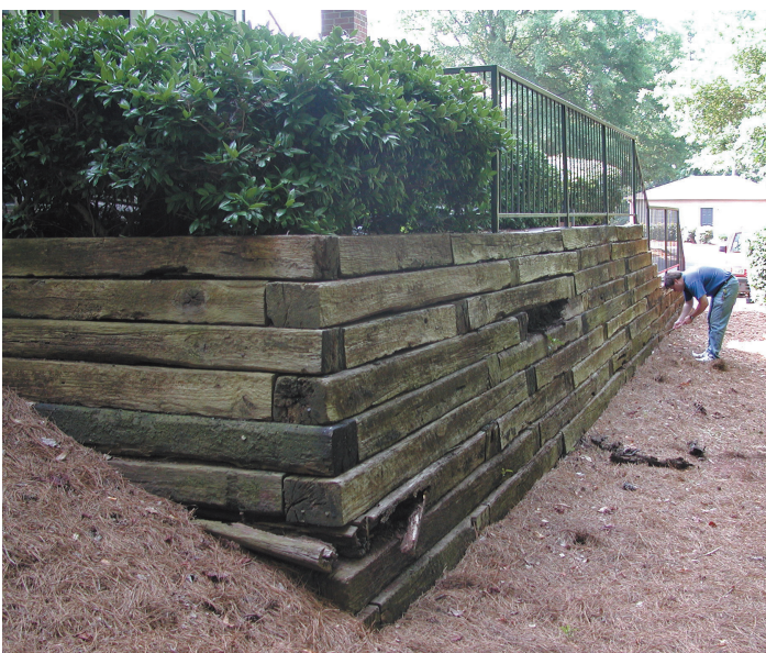
Figure 1. Formosan termites are most commonly spread when infested railroad crossties are used to build retaining walls and other structures. The presence of crossties on one's property, however, is not absolutely indicative of Formosan termite presence.
